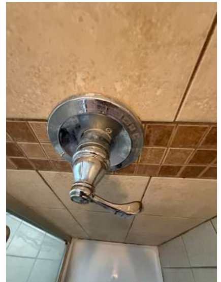
Feel around metal piece connected wall Handle is loose
