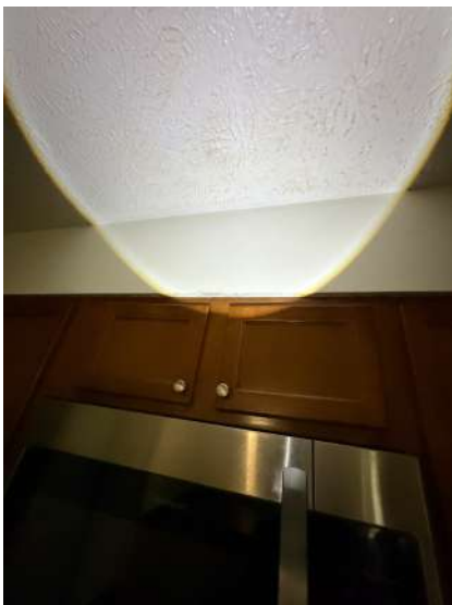
Kitchen ceiling over stove has discolored because of lack of ventilation
