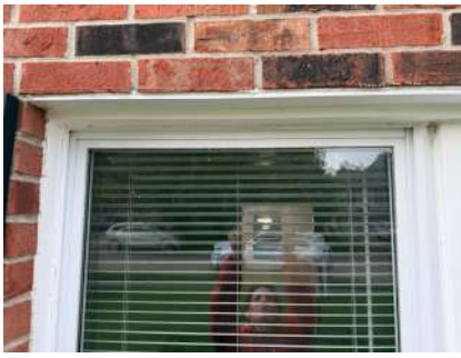
First floor left side needs to be sealed better
