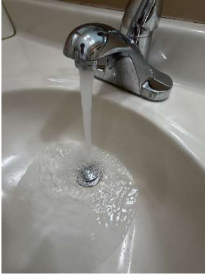
Left sink drain bubble
