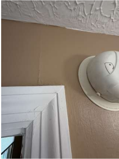
Vertical crack on inside of master bathroom
