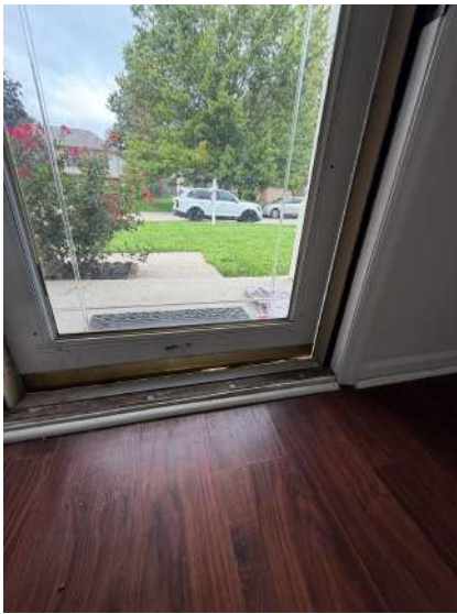
Front storm door did not securely close weatherstripping on bottom was ragged
