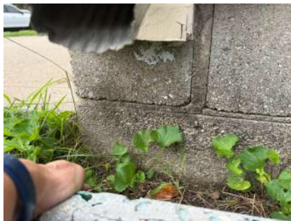
Cracks in mortar right side front
