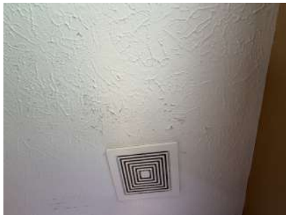
Ceiling is peeling around fan
