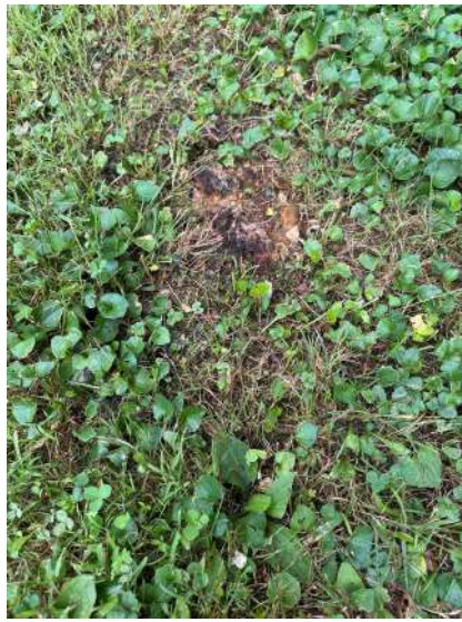
Rotting stump left side of house
