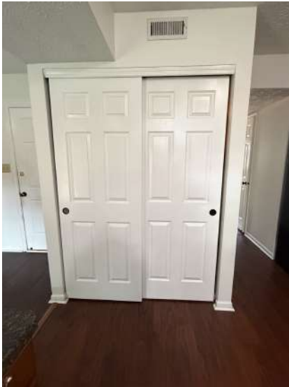
Utility closet doors were not on bottom track leaving them to swing into utilities
