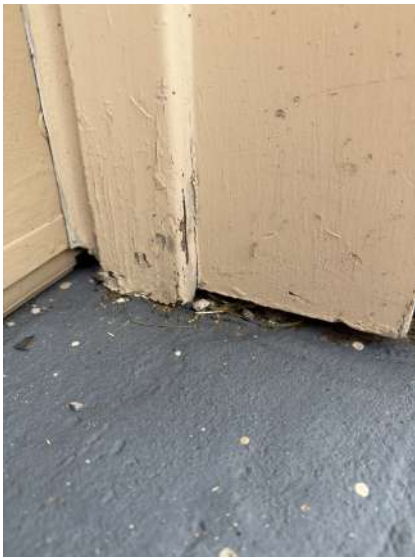
Right side, garage door, beginning to rot recommend raising the trim quote. Stop above the concrete to prevent water from entering.
