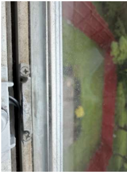
Cream room window does not lock misaligned coming off of track
