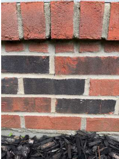
Crack And Brick under first story front window
