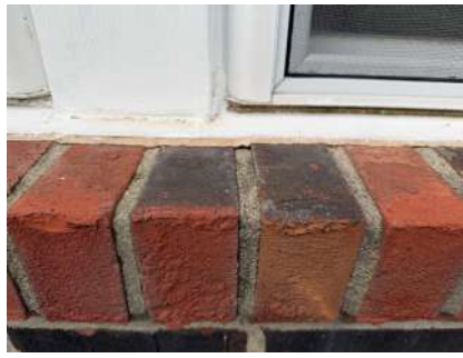
Gaps and sealant around sale first floor left side
