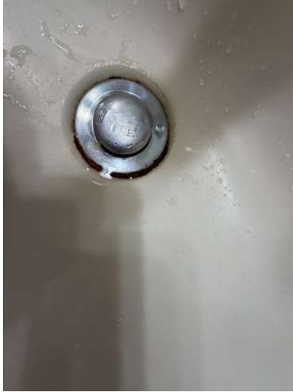
Corroded drain right side
