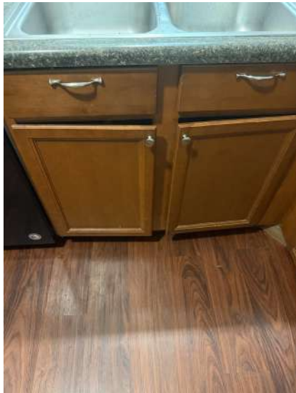
Cabinets underneath kitchen sink didn't close
