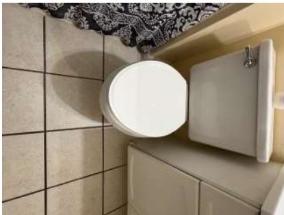
Hall bathroom toilet loose Slow drain
