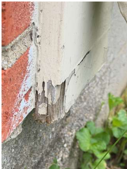
Behind front right downspout
