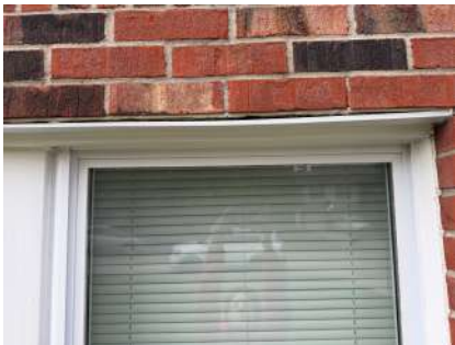
First floor left side of house vinyl trim, pulling away from lintel
