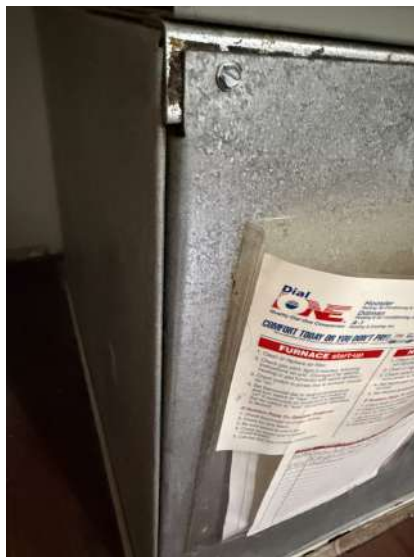
Air leaking out
