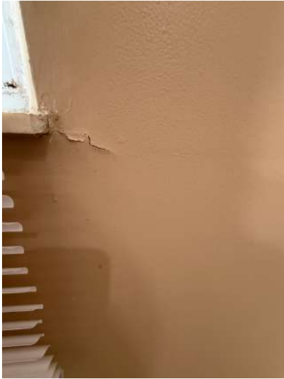
Crack on the right of master bathroom window. Most likely drywall tape.
