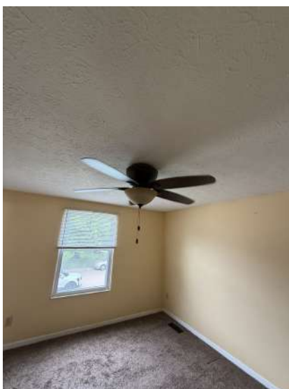
Yellow room fan was loose
