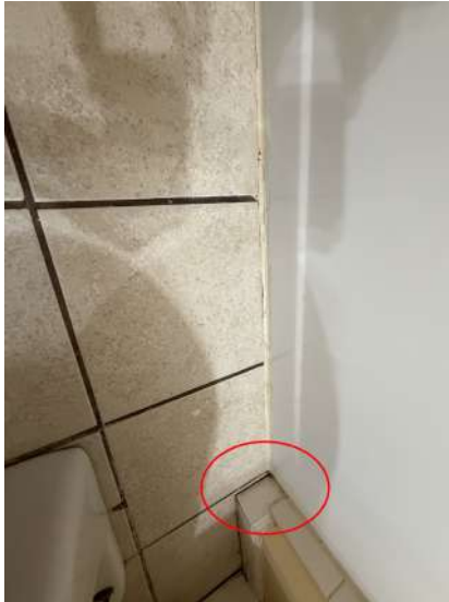
Caulk between floor and tub cracked trim next to tub
