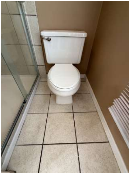
Toilet is loose and does not flush
